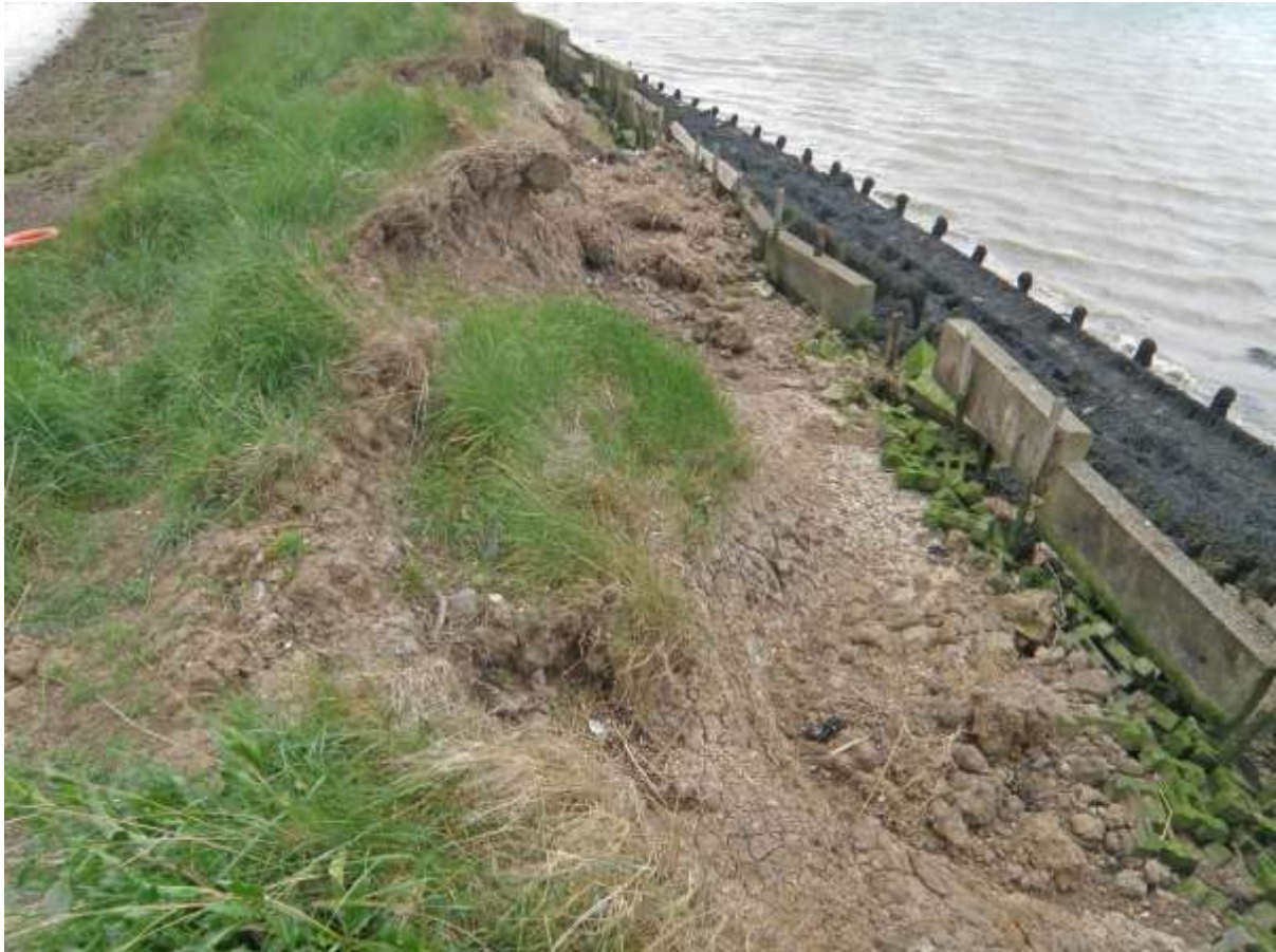
Figure 5. Erosion of the former sea wall at Trimley, Stour & Orwell Estuary, Suffolk.
