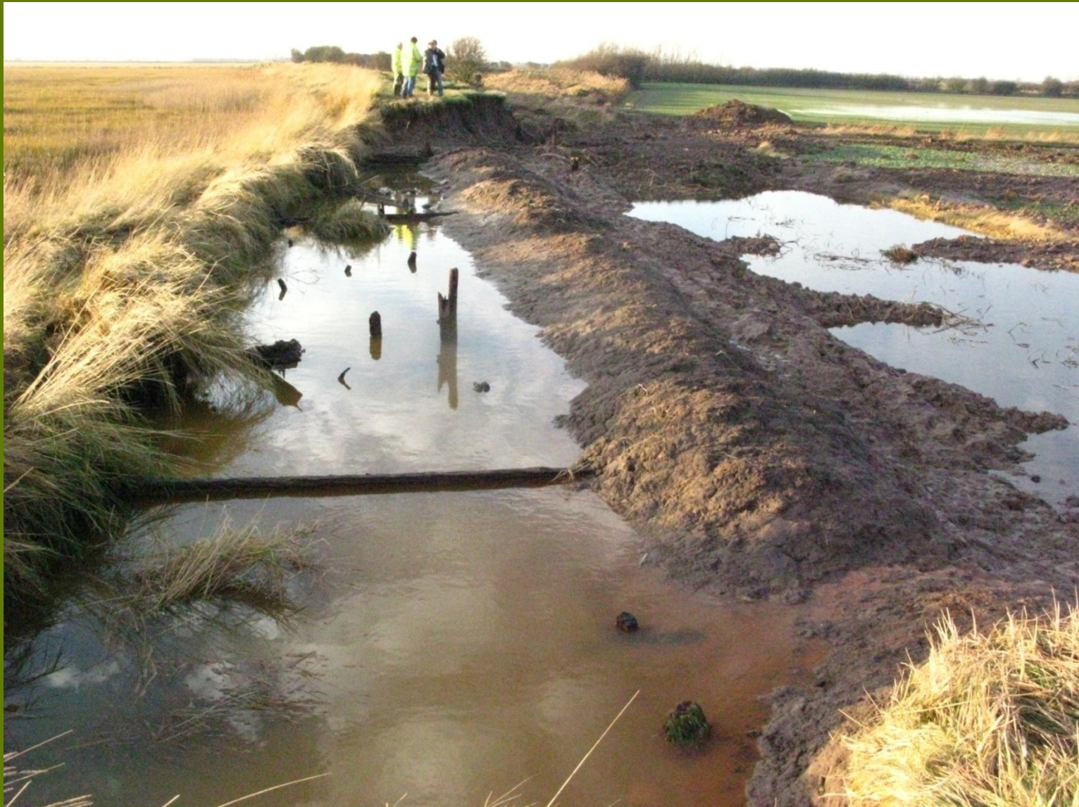
Breach of the Bank at Welwick
