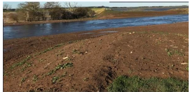
Breach site at high water
